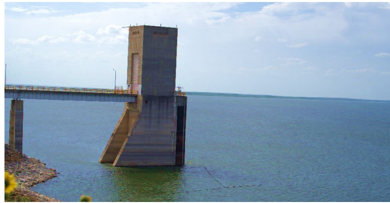
Falcon Dam plays a crucial role in the water supply for Brownsville, Texas, and the surrounding region.
