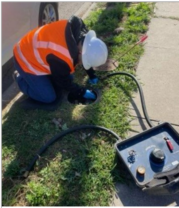
BPUB has acquired new equipment to inspect infrastructure for leaks.
